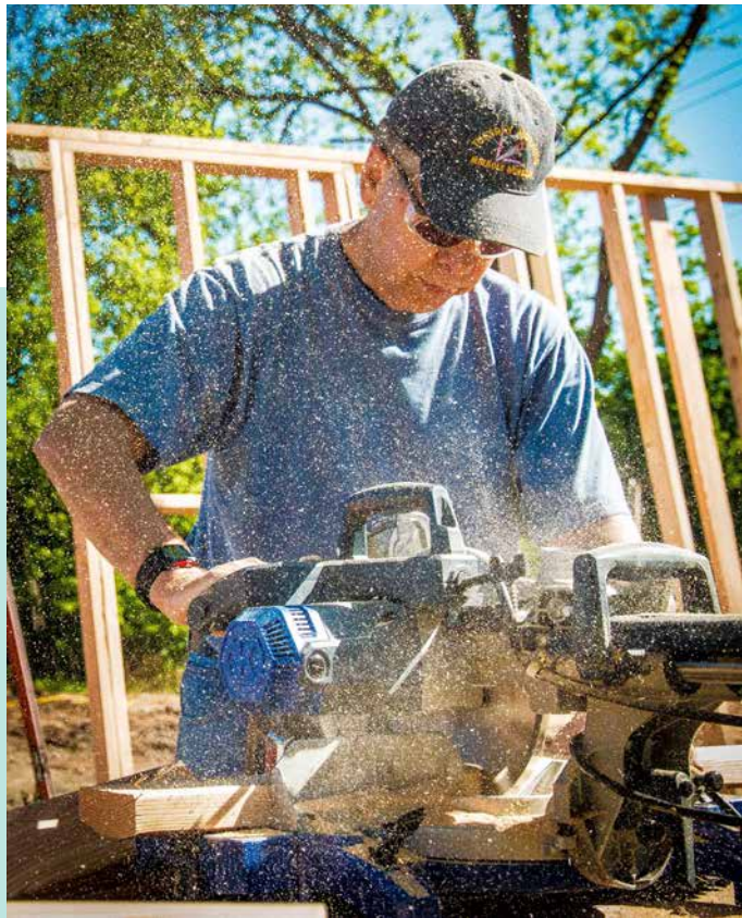
(Right) Treak Tasker and other St. Bernard volunteers move a wall into place. (Below) Sawdust flies as volunteer Dan Lubojacky gets the boards cut to size for the St. Bernard's sponsored home.
